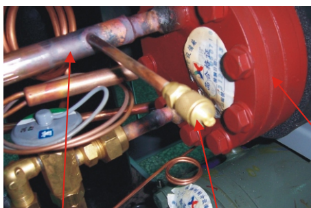
The air return pipe
