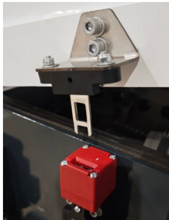
Picture 5-1: Feed Box Safety Switch Pin
