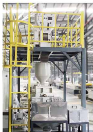
计量混合 Dosing and Mixing
